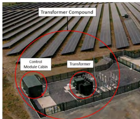
Figure 5-2 Example Photograph of UTF Transformer Compound
